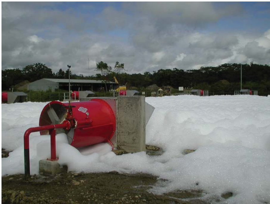
Figure 3: High Expansion Foam Discharge – Photo Courtesy of Chemguard
