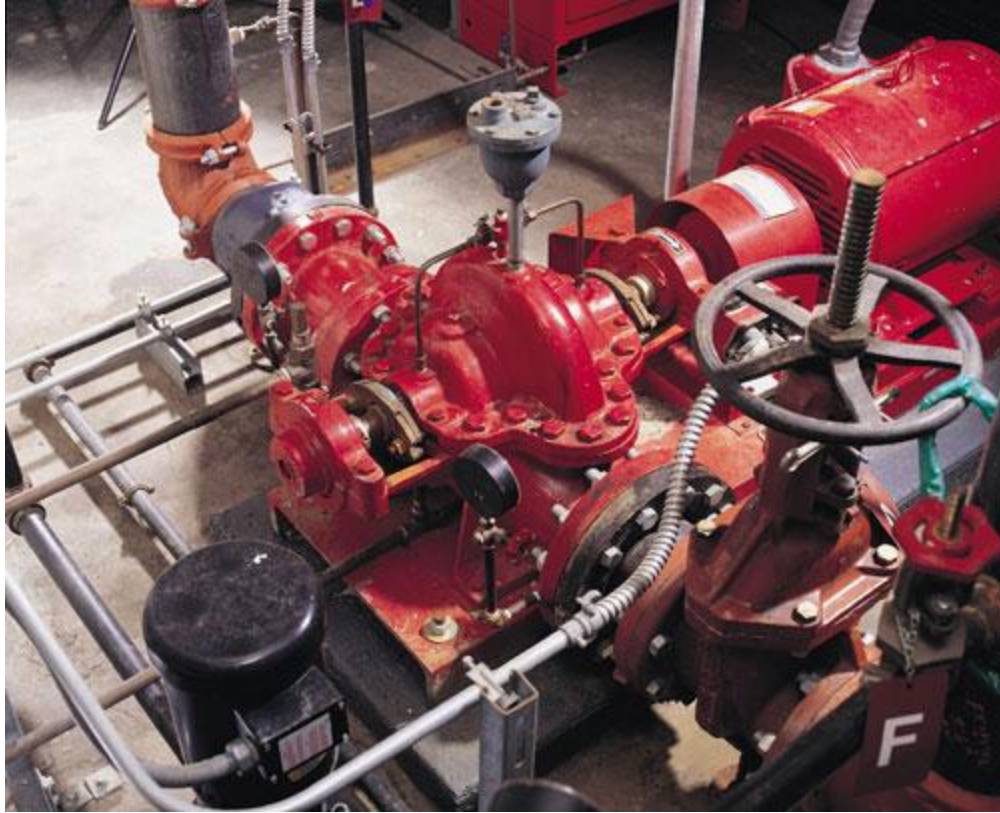
fig-3. electric pump
