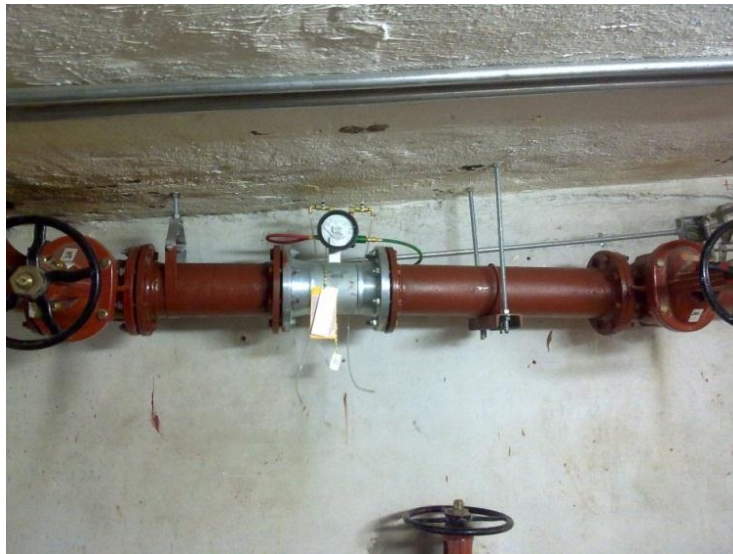
fig-17. installation of flow rate measuring device
