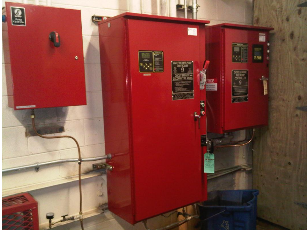
fig-5. fire pumps controllers
