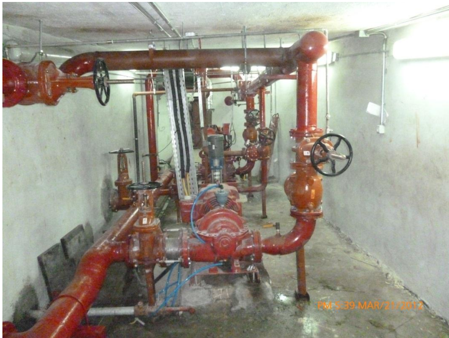
fig-8. fire fighting pump room
