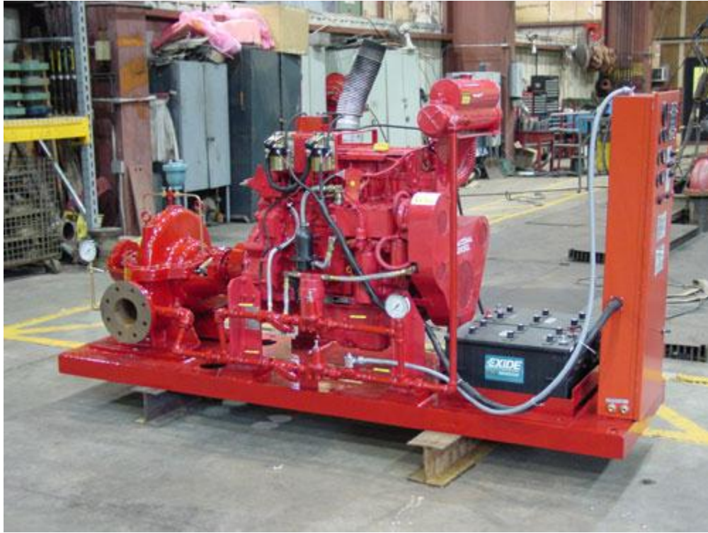
fig-2. diesel pump
